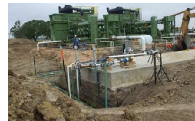
During Construction Phase: Valerus provided foundation design, engineering, construction, interconnect, the control system including emergency shutdown and 3300 Hp of compression equipment, pumps, tanks and vent system.
