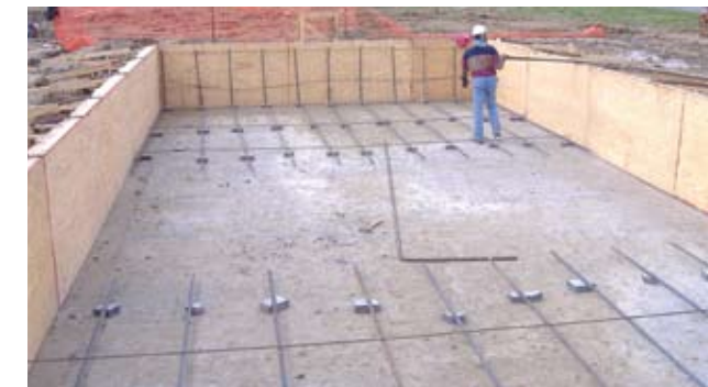
Rayne Compressor Station Expansion: Engineering Procurement Services (EPS) project during its initial construction phase. Project began with greenspace.
